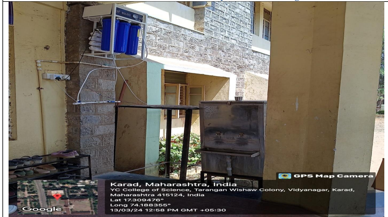
RO+ UV Water Purifier at Department of Computer Science
