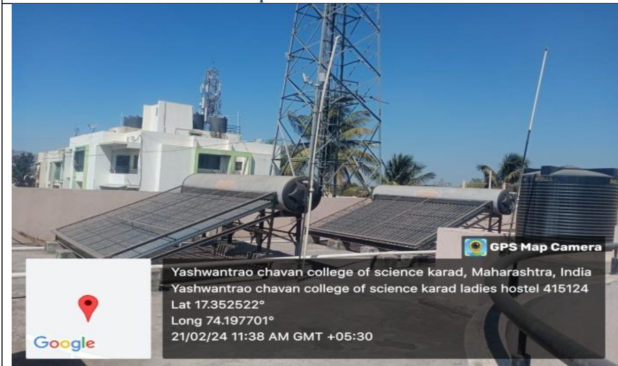
Solar panel at Women's Hostel
