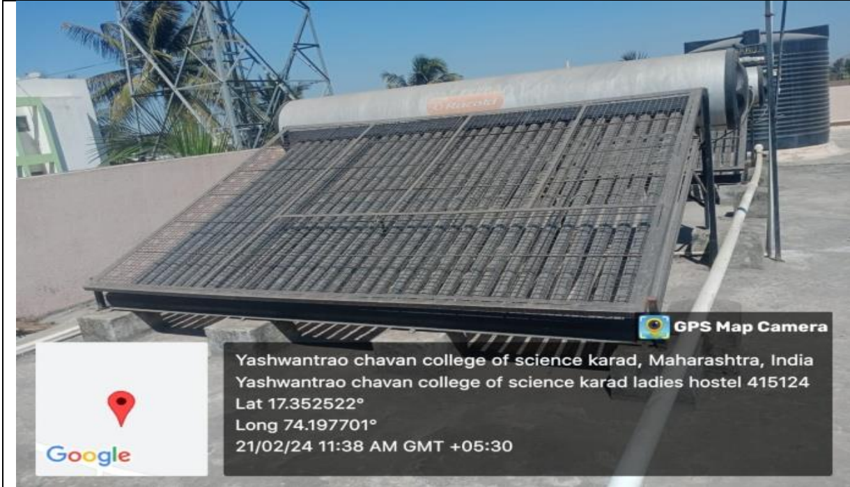
Solar panel at Women's Hostel
