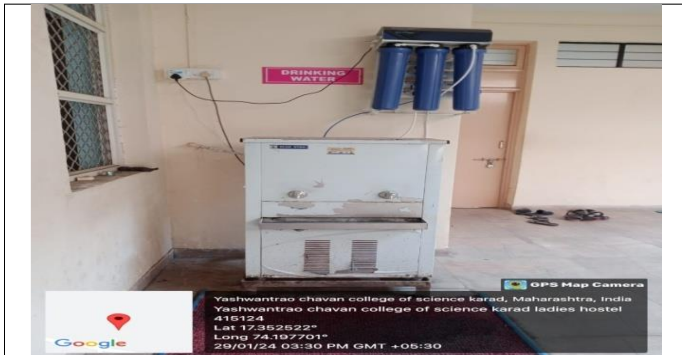
RO+ UV Water Purifier at Women's Hostel
