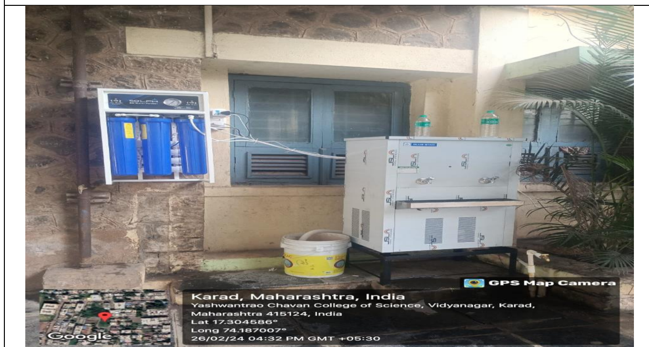
RO+ UV Water Purifier at Boy's Hostel
